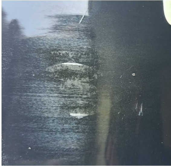
Exemplary damage of level 1 caused by impact
